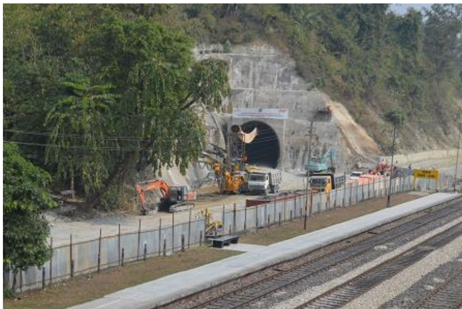
Fig. 1 - Portal location and alignment of Tunnel-1 of the 44.39 km long tracks connecting Sivok (W.B.) to Rangpo (Sikkim)
