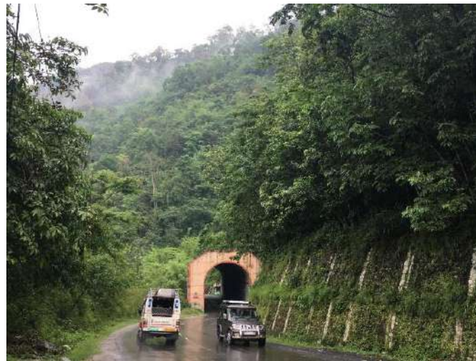
Figure 7b - Recent construction of a tunnel and retaining wall for mitigation of the Burdang landslide
