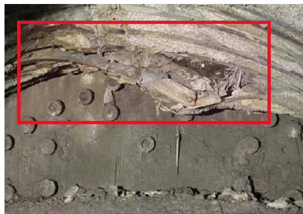
Figure 15b - Maximum deformation (within the red rectangle) occurred during grouting at the right-side crown when the injection pressure was 3.4 MPa
