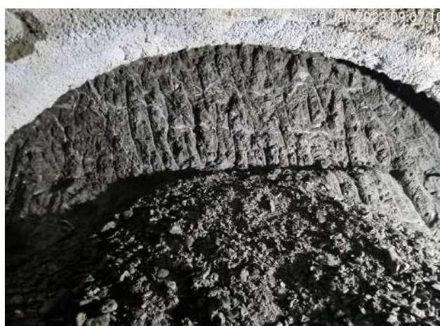
Figure 14d - Grout penetration (thick grey) lines seen at the tunnel face during the excavation
