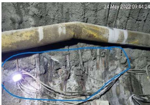
Figure 15a - The peeling of shotcrete and buckling of steel ribs. The deformation, 10 – 15cm (within the blue circle), occurred at the right-side tunnel arch during grouting with pressure at 2.9 MPa
