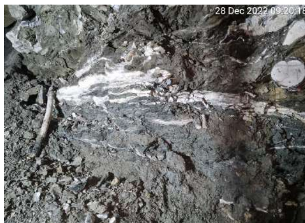
Figure 14b – Thick white lines, indicating grout penetration, observed during the excavation of collapsed material after grouting
