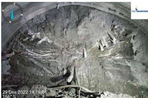
Figure 14a – Collapsed material after grouting with damaged previously installed canopy pipes.
