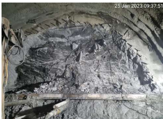
Figure 14c - In-situ claystone, after grouting with damaged previously installed canopy pipes
