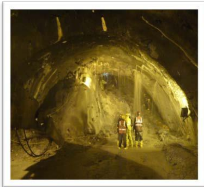
Figure 13- Heavy ingress of water
