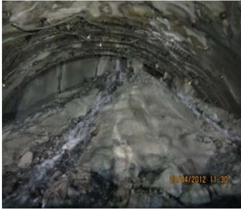
Figure 11 - Cavity at Ch. 2+045m
