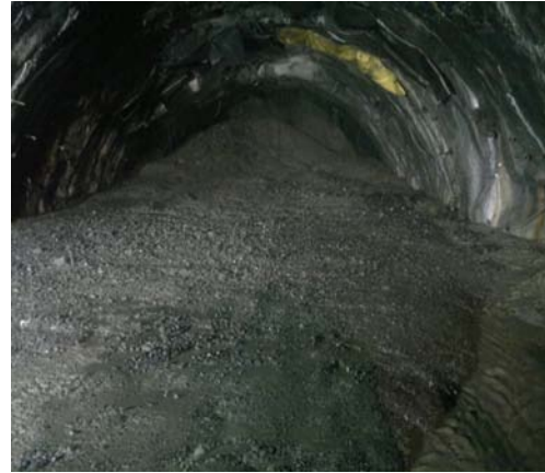
Figure 12 - Cavity at Ch. 2+077m
