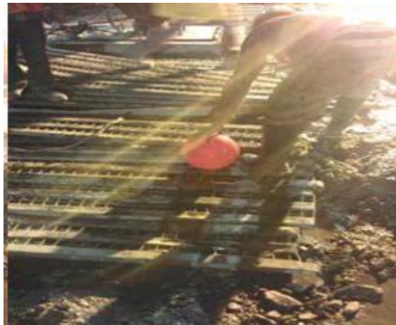
Fig. 28 - A plastic ball is placed in tremie pipe to prevent mixing and concrete segregation
