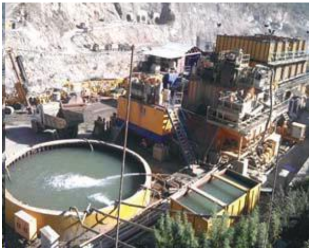
Fig. 16 - Bentonite mixing plant
