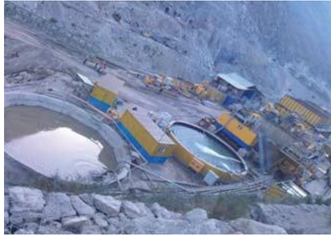
Fig. 20 - Dykes for storage of bentonite
