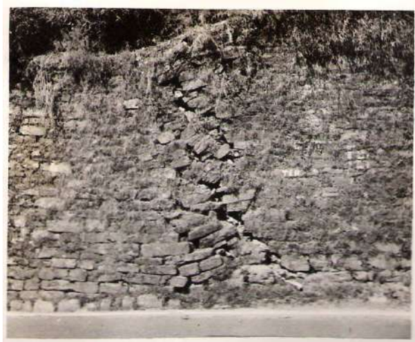
Fig. 5- Uneven settlement of boundary wall of railway building
