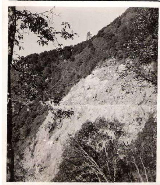
Fig. 4 - Slope failure due to widening of road
