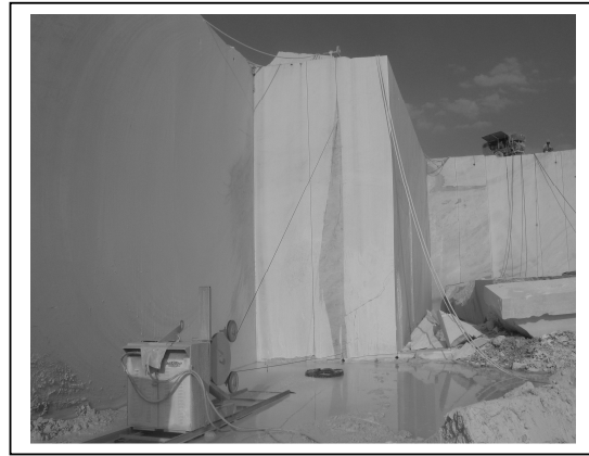
Fig.2 – Vertical cut with diamond wire saw (variable speed) at Pit no. 40 in medium dolomitic
