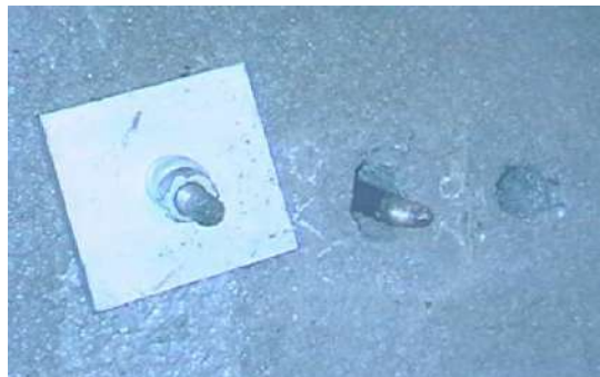
Fig. 3 - Failure of thread portion of 12m long Tor steel rock bolts during efficacy test
