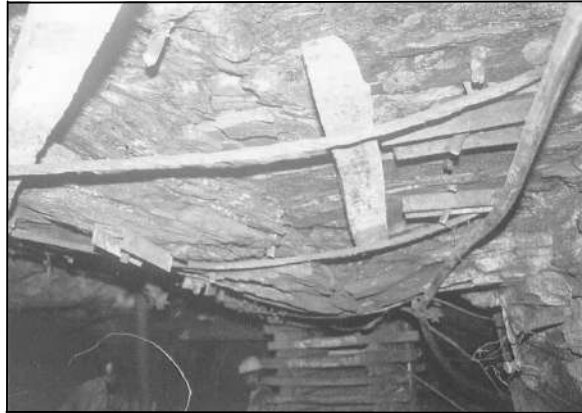
Fig. 3 – Location 116 LS-2D: Sagging and compressional crack developed in the roof strata resulted into ‘Gutter Roof’ in 116 level
