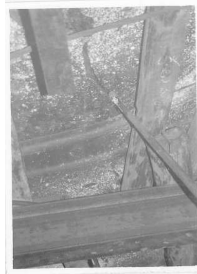
Fig. 8 – Failure of roof associated with cleats and bend in the W-strap support
