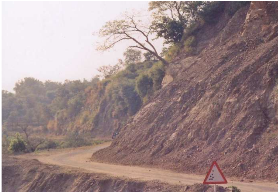
Fig. 2 – Slope failure because of toe-cutting for construction of highway
