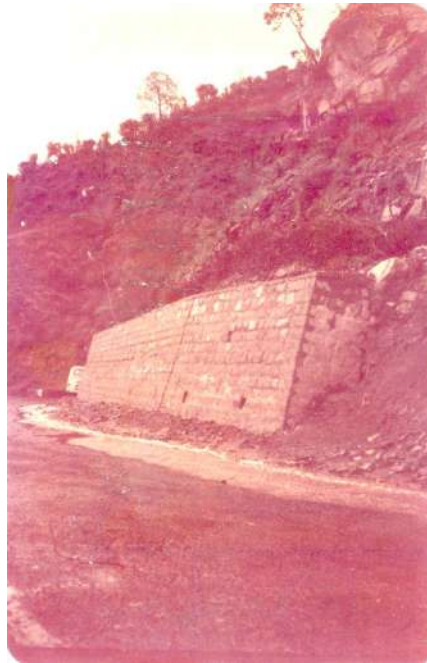
Fig. 1 – Rain water flowing on the road in the absence of drainage facility. A breast wall is there on hill side
