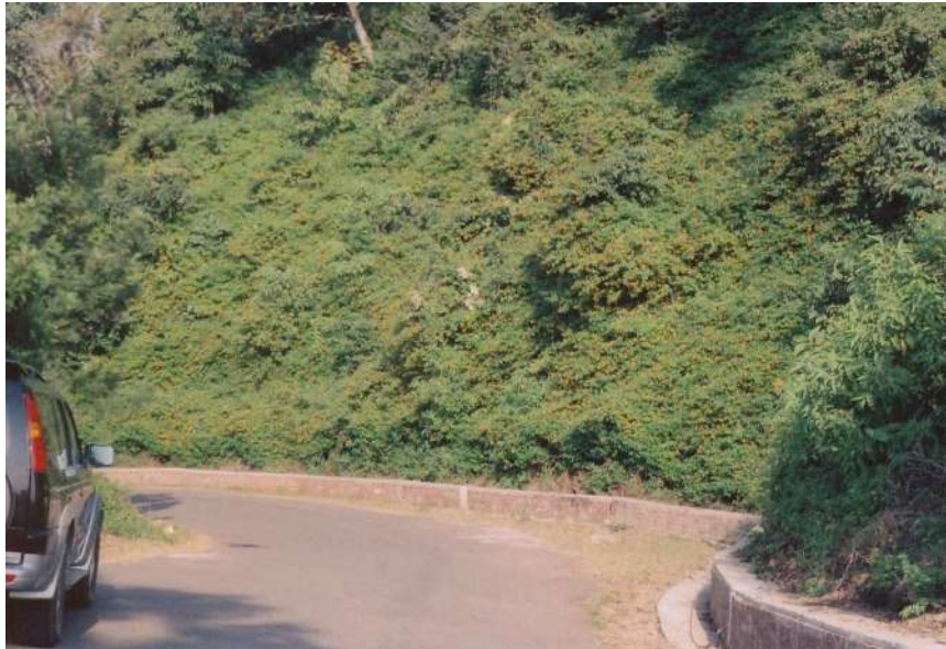
Fig. 7 – A view of the recently constructed side drain at the proposed location (RD 24000m)
