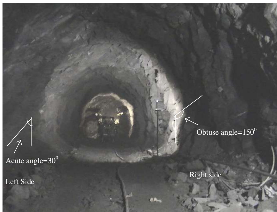
Fig. 3 - Penstock tunnel with acute joint orientation (Left side) and obtuse joint orientation (Right side) with respect to the tunnel profile
