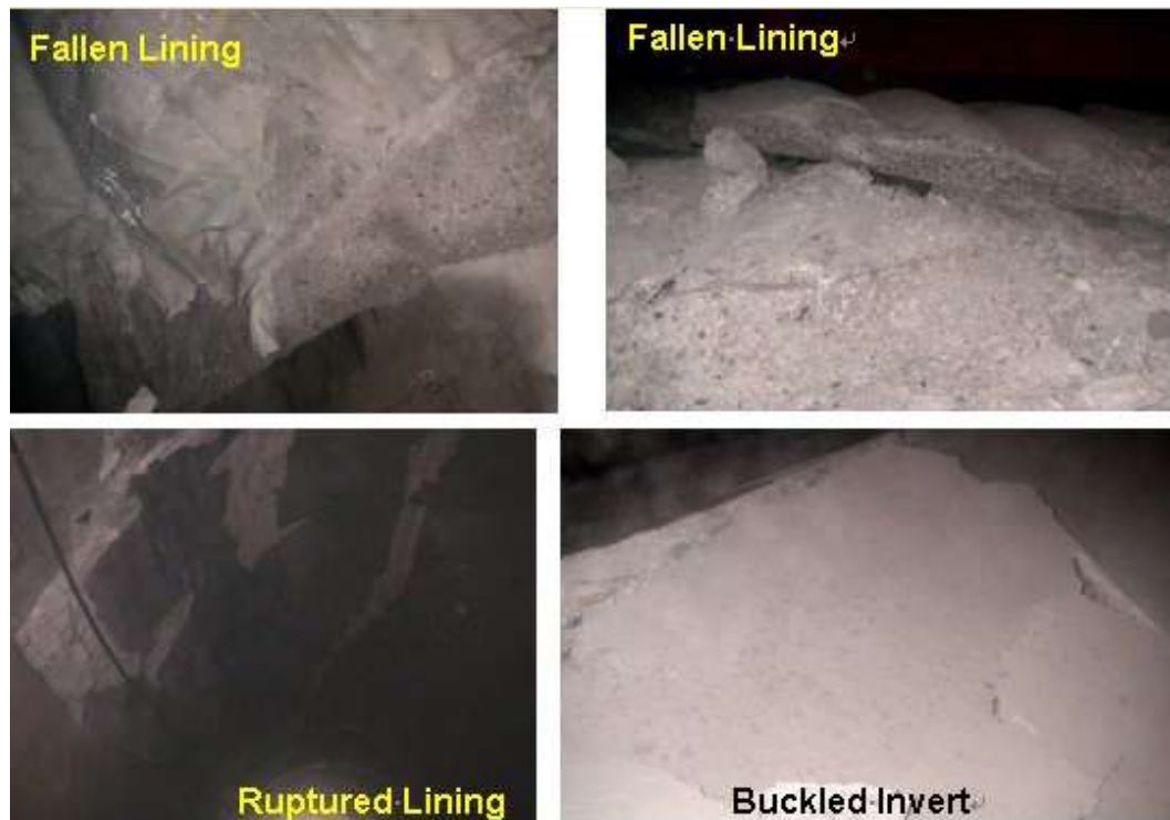
Figure 23. Views of earthquake damage at Longxi (Longqi) Tunnel
