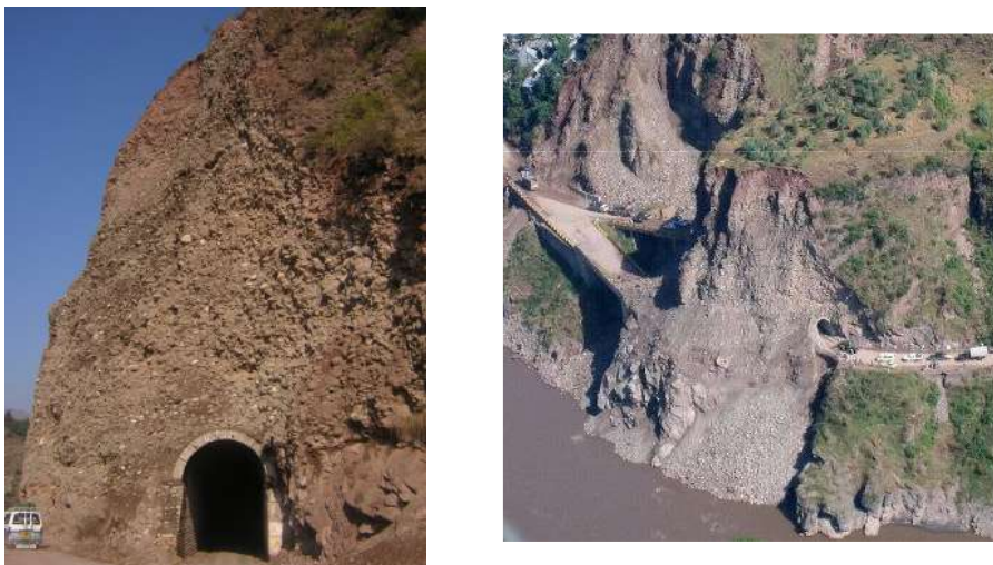
Fig. 20 - Lightly damaged roadway tunnel
