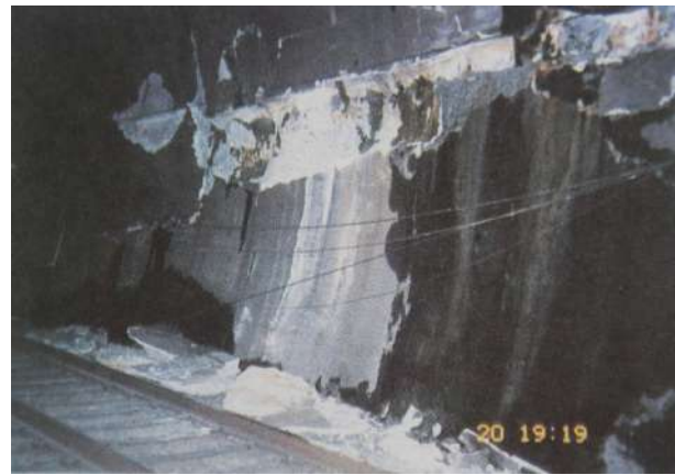
(b) Side wall spalling
