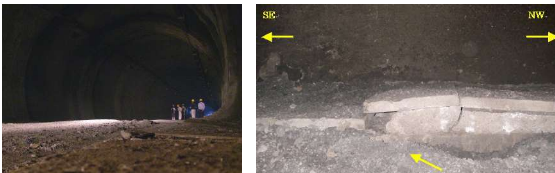
Fig. 22 - Views of repaired damaged section of the tunnel near the Zipingpu dam
