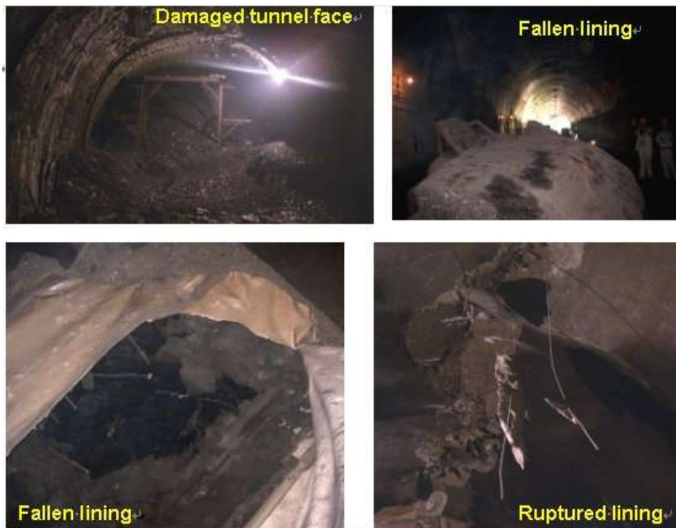
Figure 24. Views of damage at Jiujiaya Tunnel
