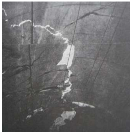
(a) Cracking in the roof
