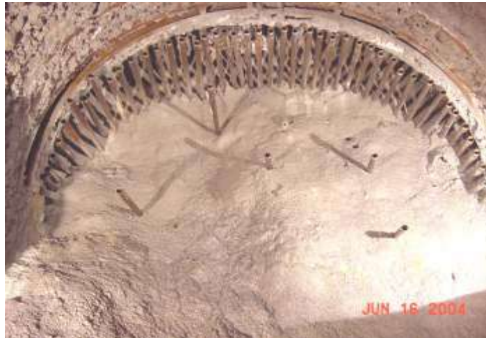
Fig. 2 - A view of forepole umbrella and drainage holes at the HRT face in AGO reach
