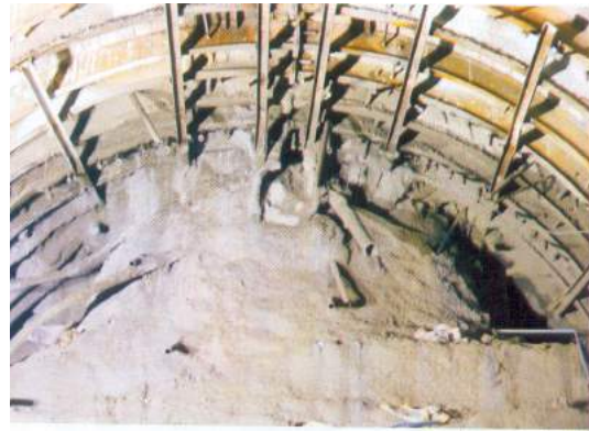
Fig. 6: Treatment of collapse in diverted alignment
