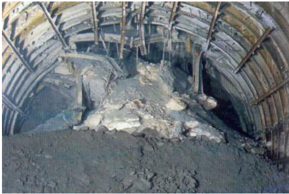
Fig. 5: Collapse in diverted alignment
