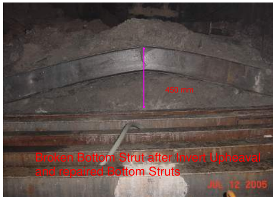
Fig. 10: Broken/replaced invert struts
