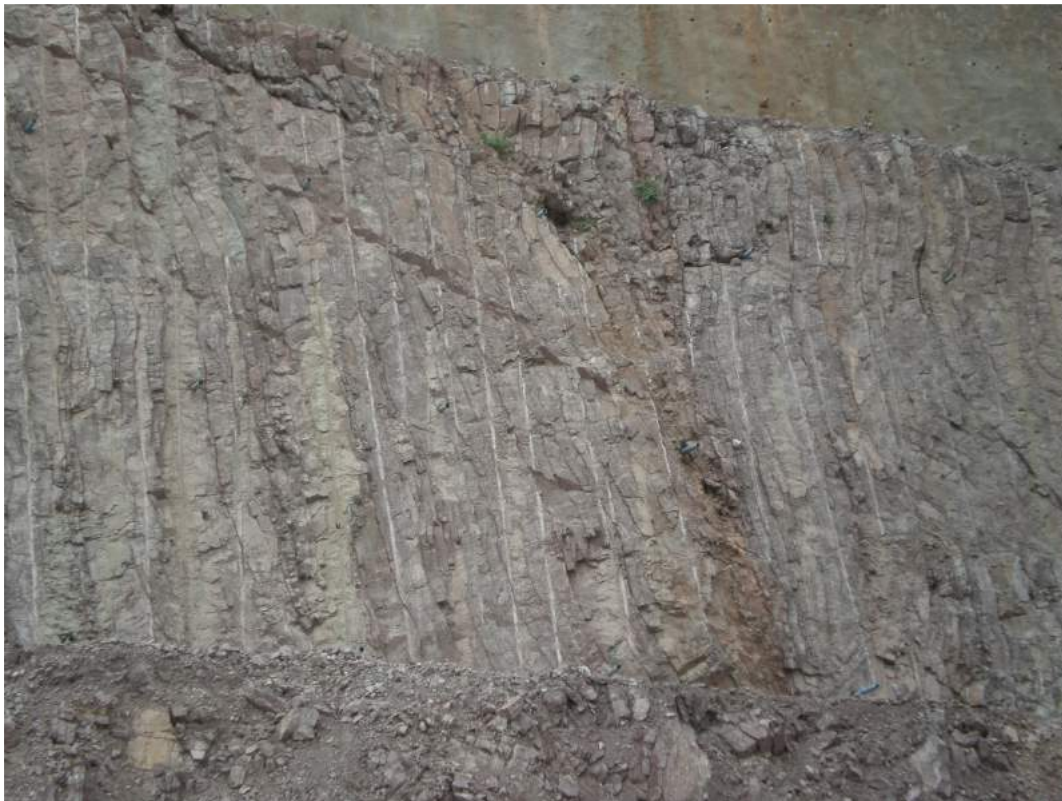
Fig. 4: Photographs showing drill holes marks after pre-split blast in approach channel area
