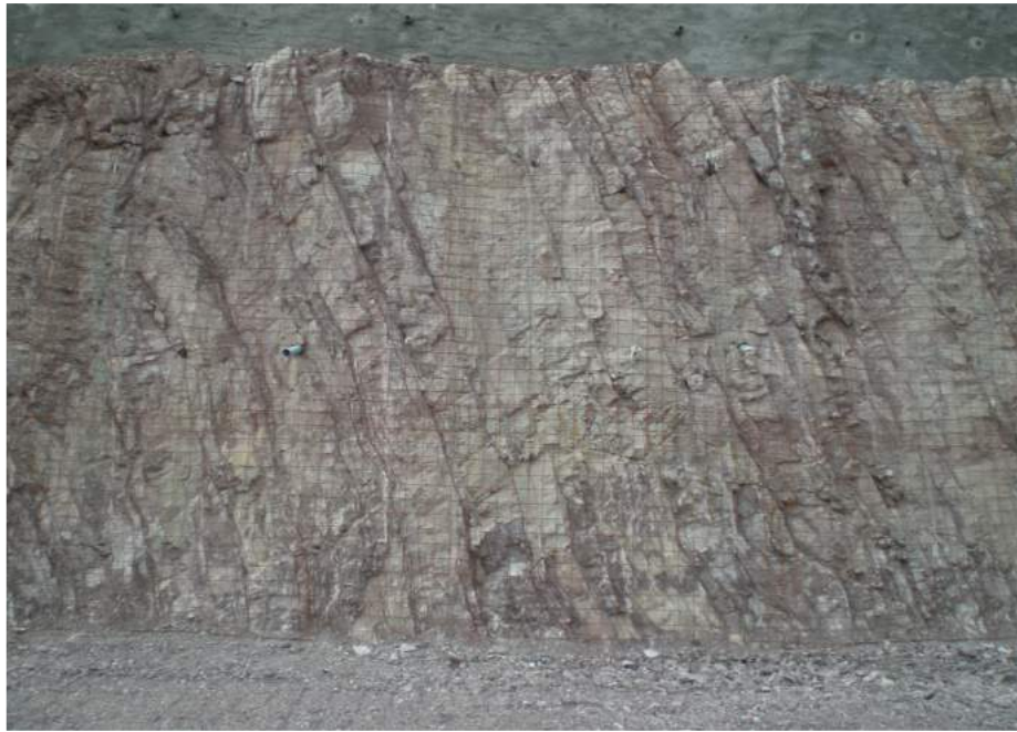
Fig. 7: Photograph showing improvement in pre-split blast results at crest portion of bench
