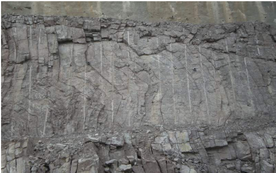
Fig 5: Photographs showing damage in the crest of the benches due to production blasts
