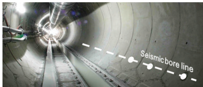
Fig. 4 -Layout of seismic holes through grouting and lifting inserts of precast segments
