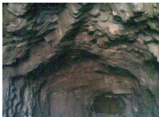
Fig. 3b - Overbreak in portal area
