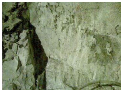
Fig. 6b - Wedge failure on wall
