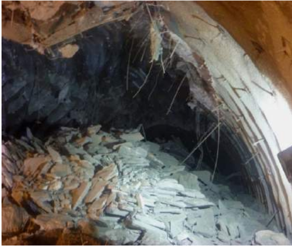
Fig.4 - Roof collapse at Ch. 7+210.89m, North portal
