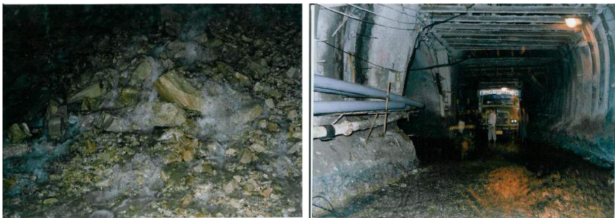
(a) (b) Figure 4: Water coming from the tunnel face and flooded the tunnel floor
