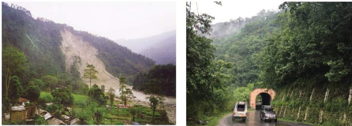
Figs. 7 a & b - The Burdang slide adjacent to the river Tista in Sikkim and the recent construction of a tunnel and retaining wall for mitigation of the landslide
