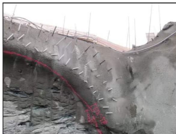
Fig. 15 Principle of combined RRS and spiling bolts (NPRA 2010) (left), spiling bolts and sprayed concrete in a tunnel in Norway (right)
