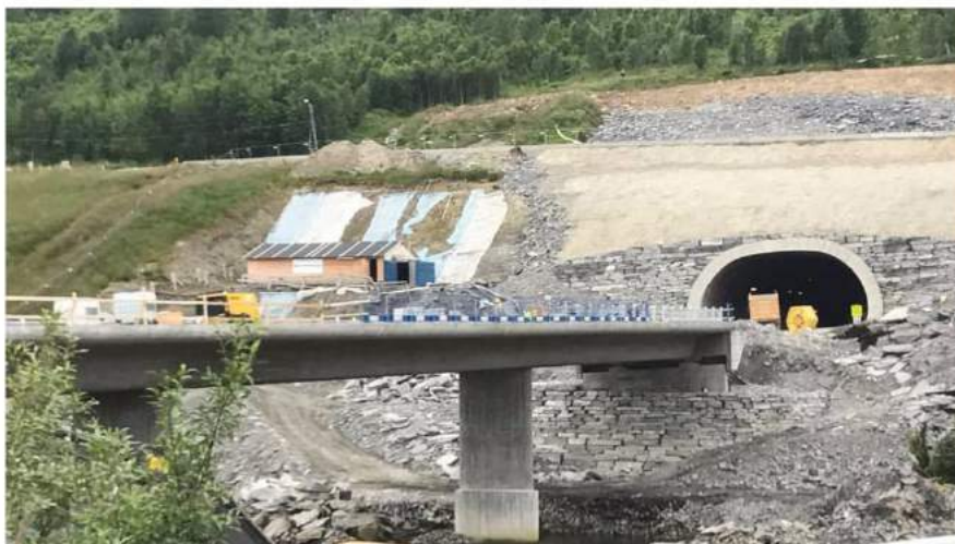
Fig. 13 - The entrance to Nordnestunnel from the Mandalen side (Photo: Jan Arild Hansen)
