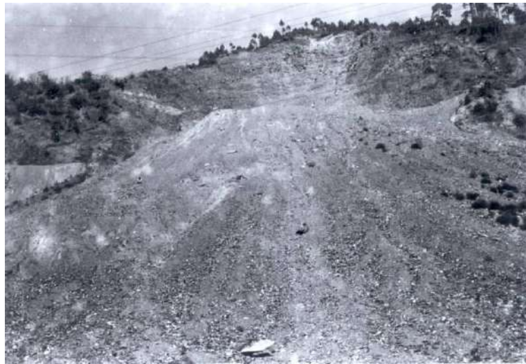
Fig. 1 - Panoramic view of problematic slope at Matli site
