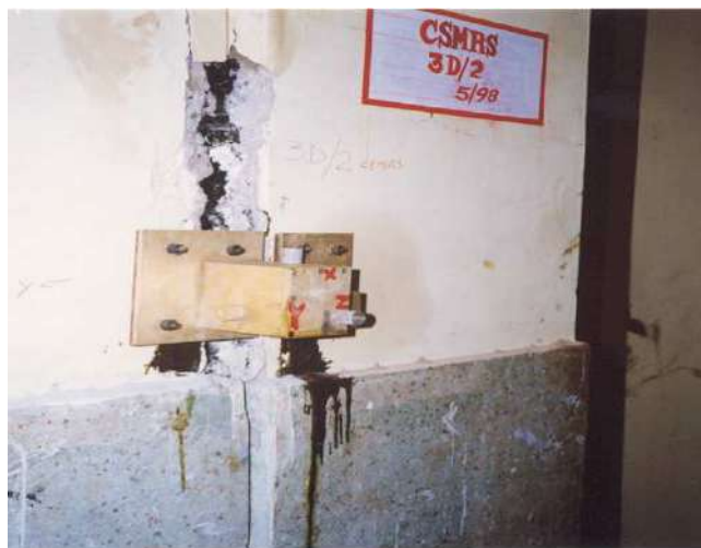
Fig. 4: Crack and Crack Monitor Near Lift of Powerhouse
